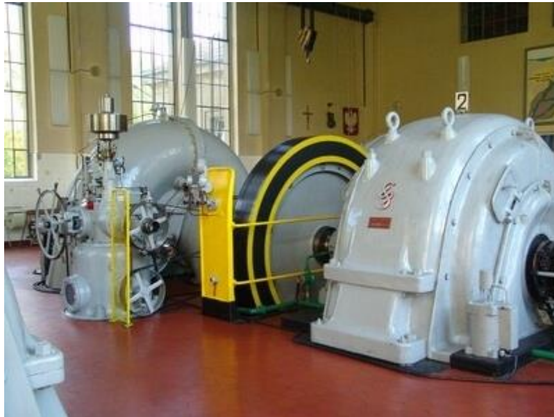
Fig.II.4. First flywheel energy storage facility in Europe (Ireland).
