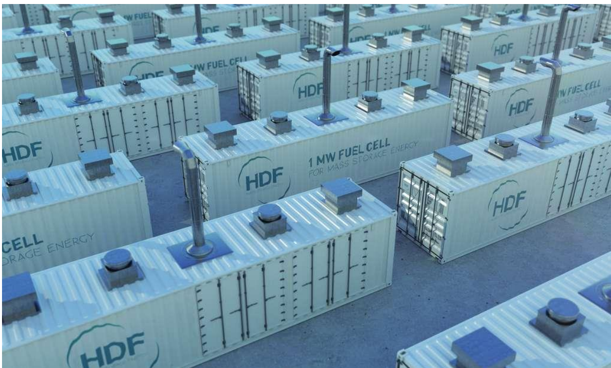
Fig.II.3. The world's largest electric storage battery is being installed in Guyana (solar electricity is stored in the form of compressed gas in bottles stacked inside 12-meter-long containers).
