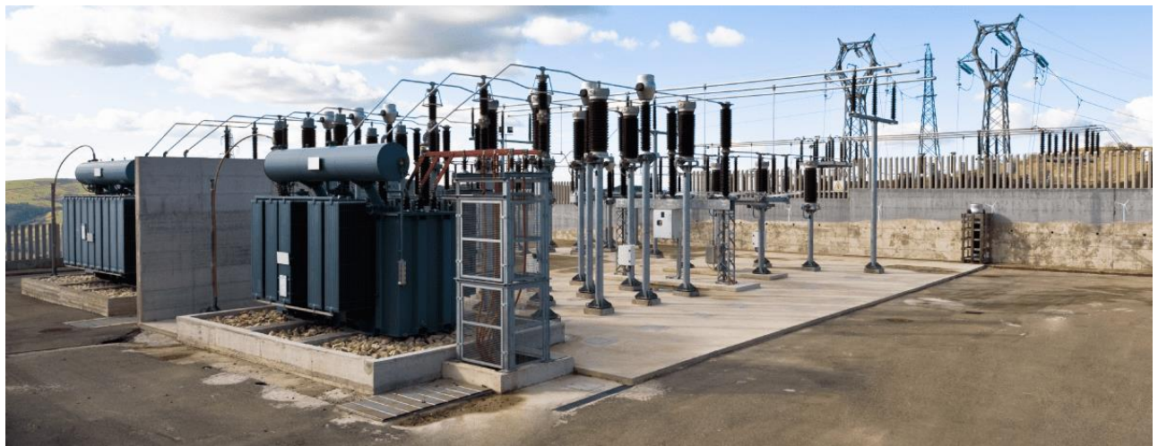
Fig.2.5: high voltage substation
