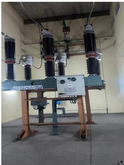
Oil circuit breaker
