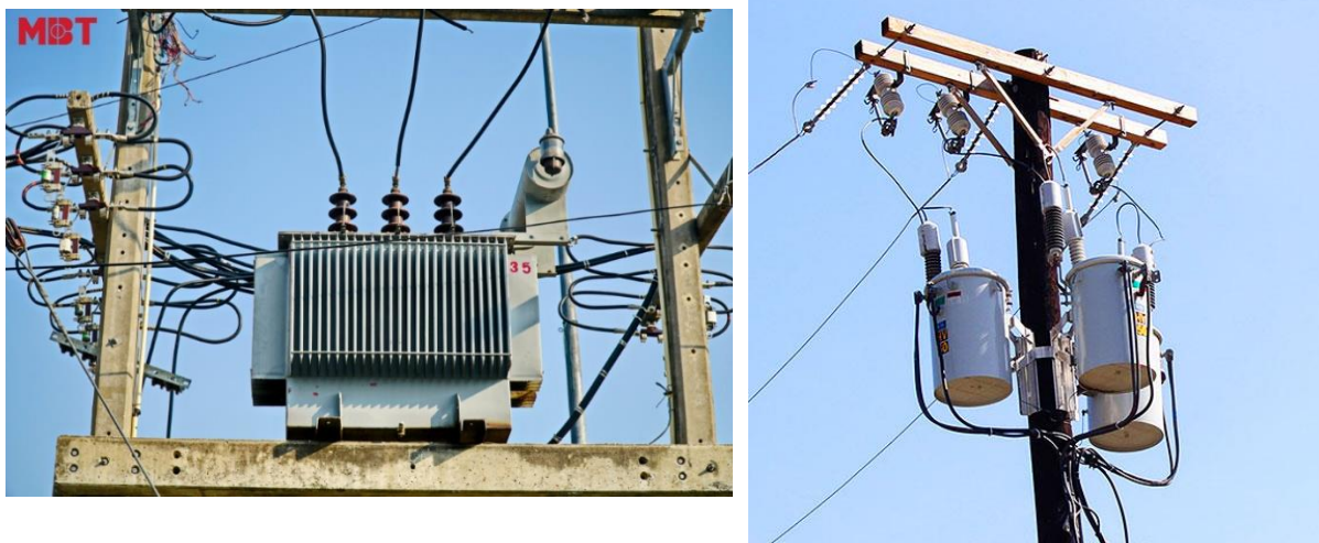
Fig. 4.10: conventional pole mount transformers
